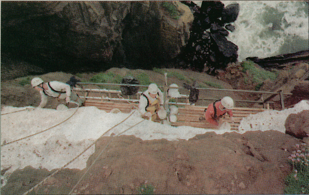
Workers abseiled to a platform to paint the 'geological timetable' rocks at Siccar.
